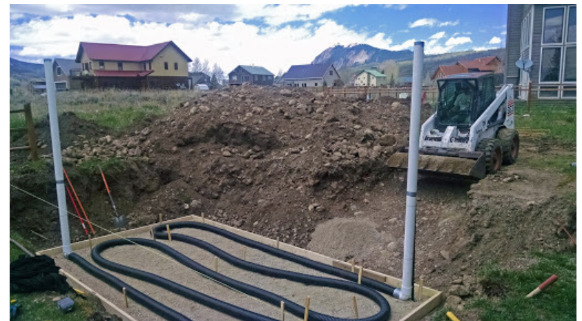
Above: Underground heat exchange tubing for a bioshelter heating system
